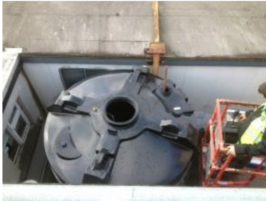
One of 3 (1000 litre) Tanks we installed.
