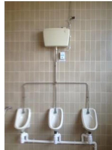
Urinals making use of the rainwater
